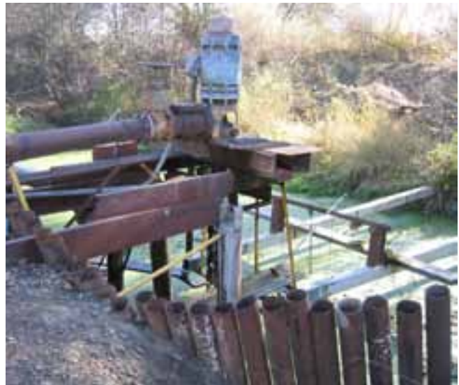
The water well and pump/irrigation ditch provide water to the site.
